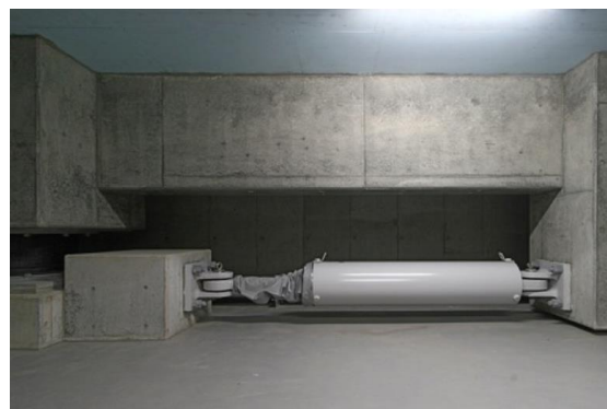
Oil damper mellem fundamenter
